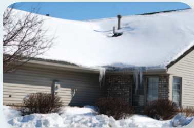
Ice dams, before removal.
